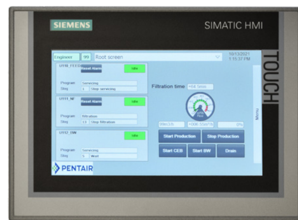
Siemens Main Control Panel.
