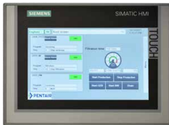
Siemens Main Control Panel.
